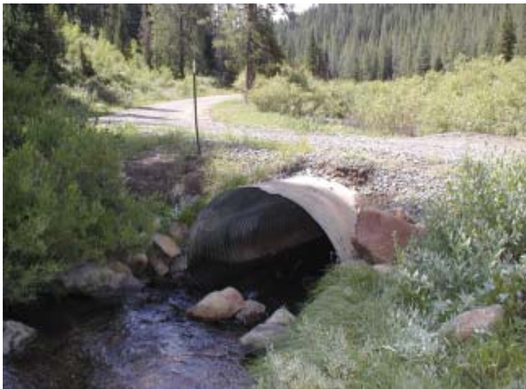
A properly sized and placed culvert will handle 50 year flood events and allow safe fish passage.
