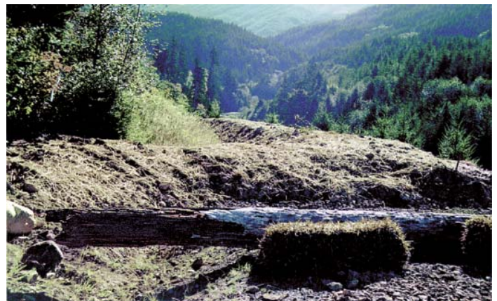
This road has been ripped and seeded, and access blocked with logs.
